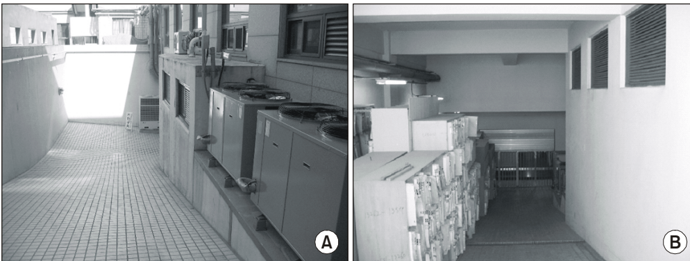
Fig. 4. Positions of air inlets and outlets. A: position of air inlets, B: position of air outlets.
